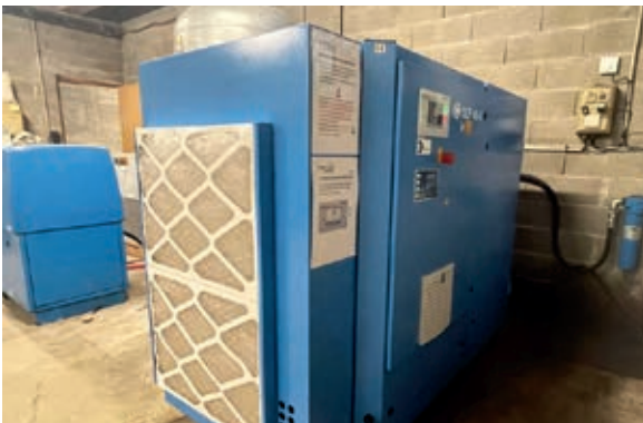
New variable speed compressor installed in Bozouls.
